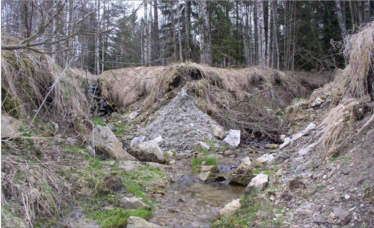
Fig. 162. Erosion and its consequences. In unstable subsoil, artificially deepened channels with a depth and width of 0.5 m erode quickly into a gully up to 2 m deep (Vyšenský potok stream 2005, water level at normal flow rate). Coarse stones, if present, remains in place.
