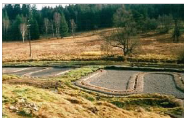
Fig. 172. The construction of rearing and reproduction features. SRRF – Blanice NNR – a layer of enriched soil with turf is visible along the future route.
