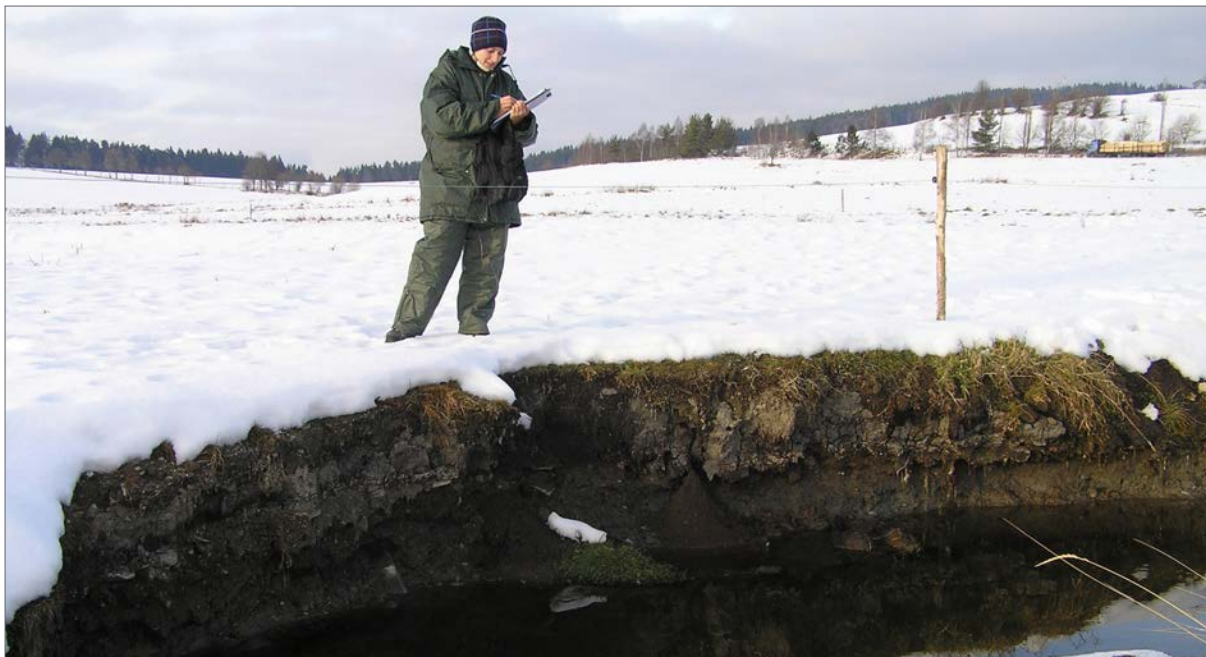
Fig. 255. State of the banks in December 2005, when massive sand deposits into the main Blanice stream had already been recorded. As a solution, growing fascine bundles with gravel were recommended.
