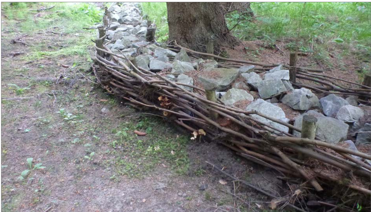
Fig. 184. A dam formed by a double willow fence filled with quarry stone. At higher water levels, the water partially flows around the dam, partially through it. Both the fine-grained and coarse-grained suspended solids are trapped in front of the dam.
