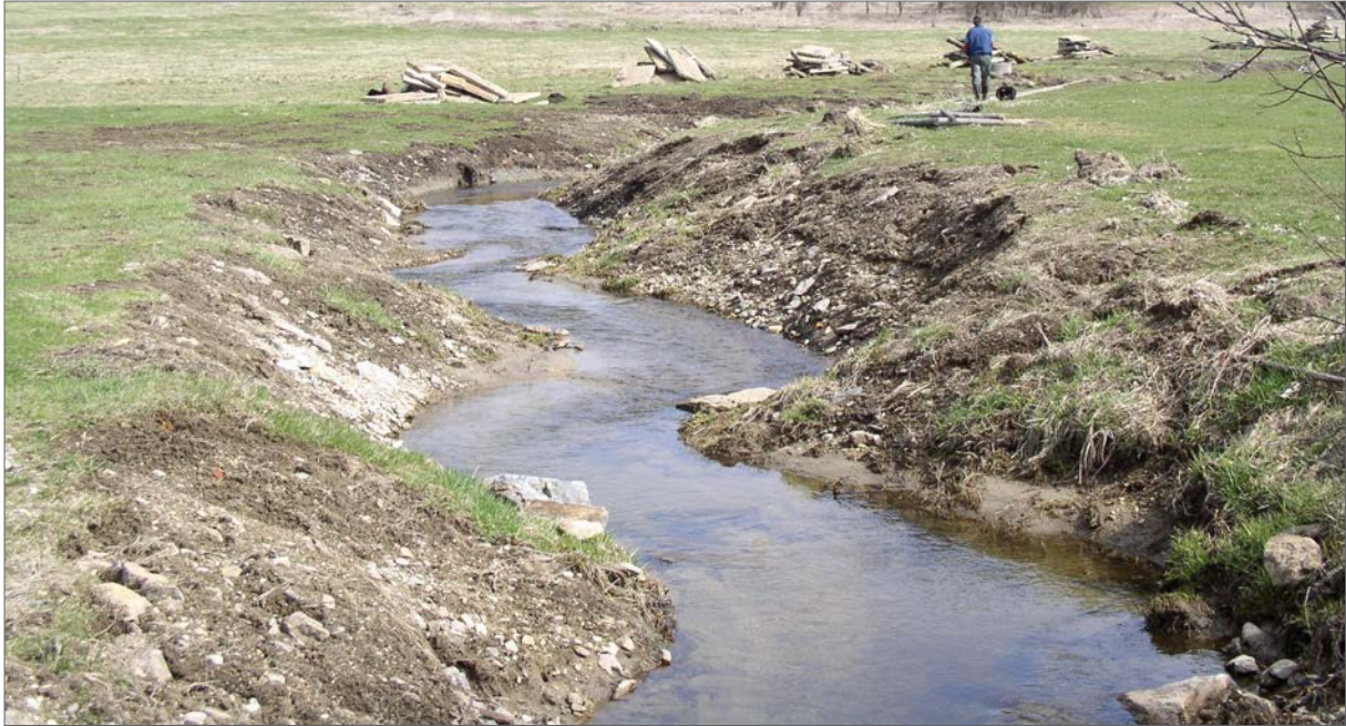
Fig. 252. In November 2004, partial riverbed revitalization was carried out – the concrete fortifications pulled out and meanders marked.
