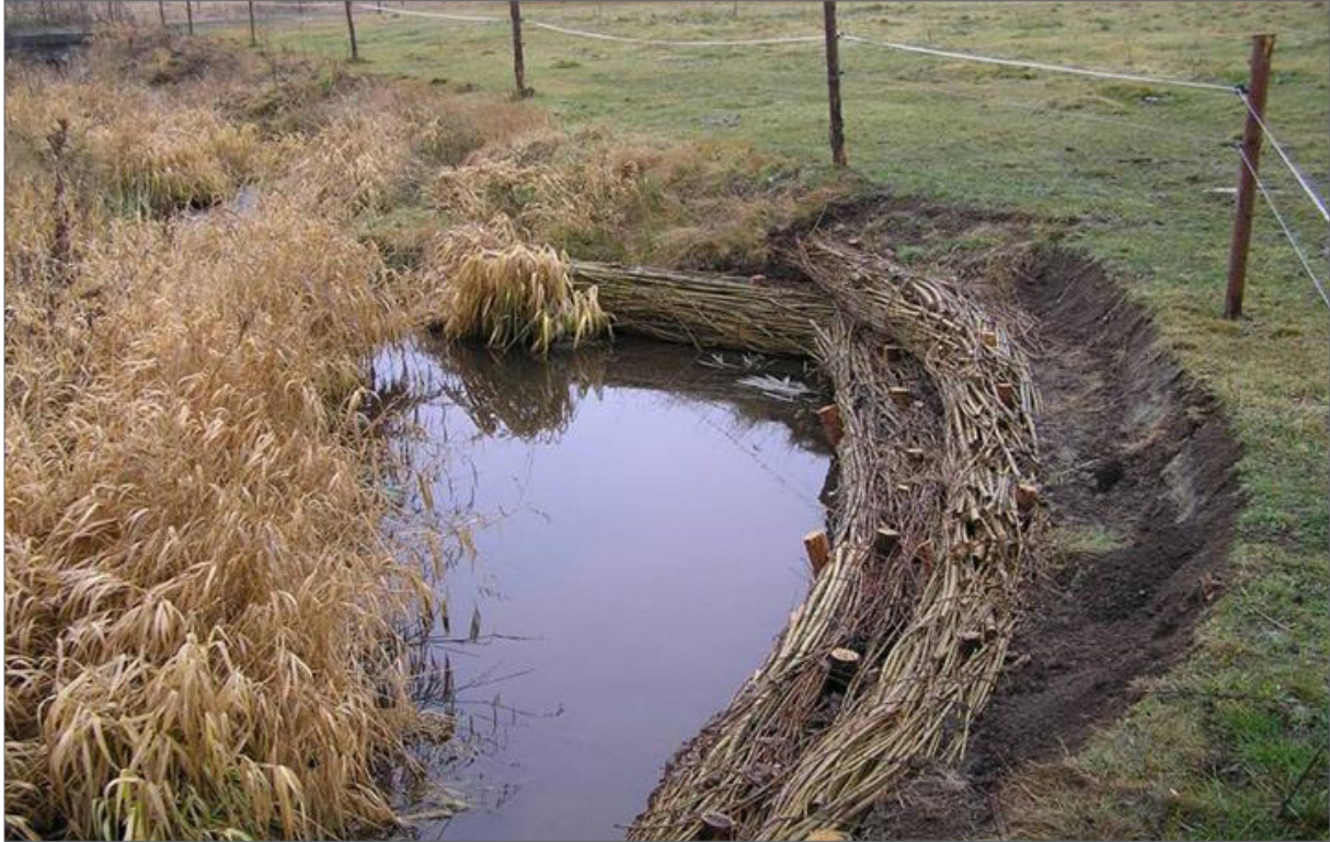
Fig. 257. Installation of a larger number of growing fascine bundles with gravel into the stream according to the project of Vejmelková and Simon (2006), carried out in November 2006 by stream manager.
