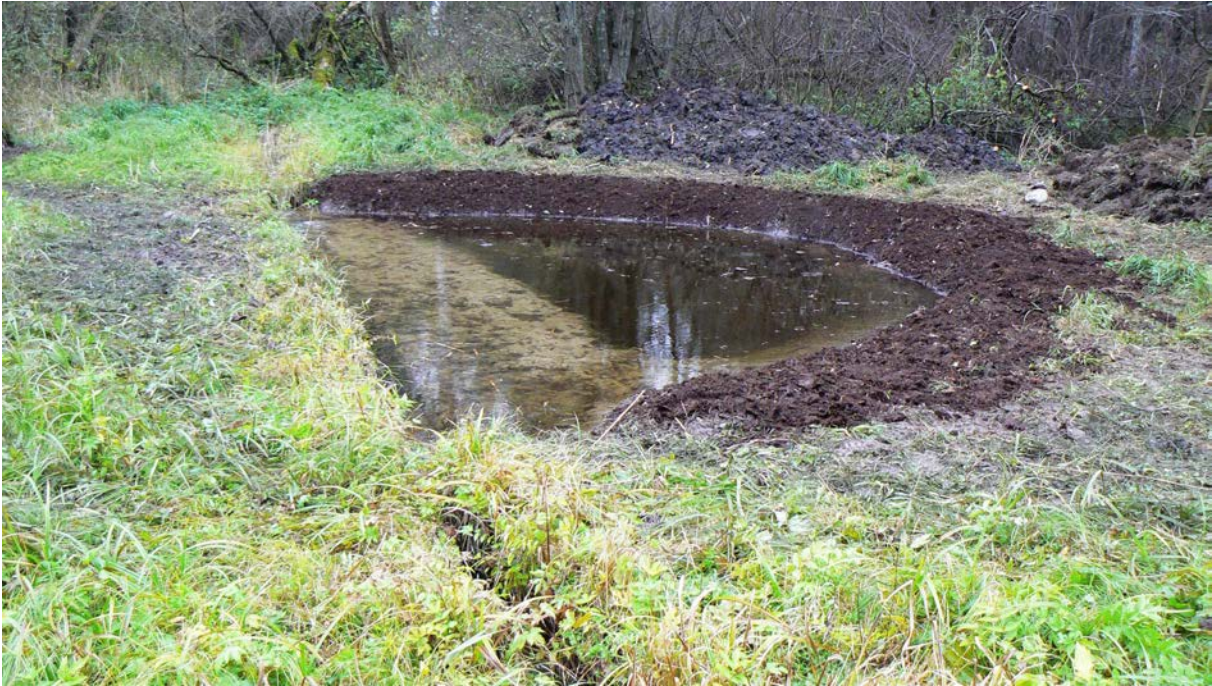
Fig. 221. Example of a side pool. The flow pool in the Zlatý potok stream catchment (ZRRF) with a combined function; it was built as an experimental-model feature to test expected functions. Pool immediately after excavation in 2010.
