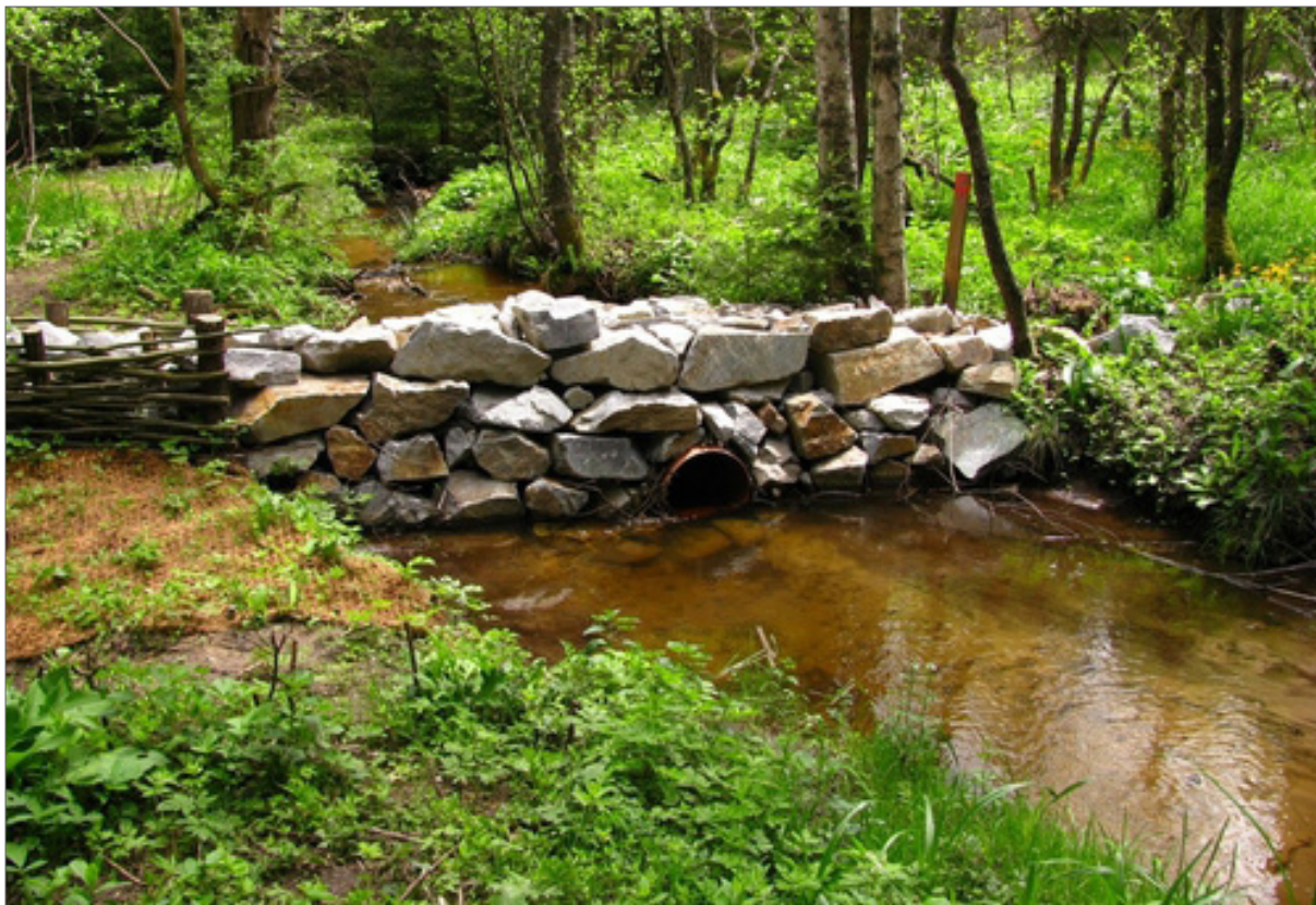
Fig. 189. Technical implementation of measures on Luční potok stream in the Zlatý potok stream catchment. Spill just after completion of construction (a plastic pipe carrying the entire normal flow and use of coconut mats is visible).
