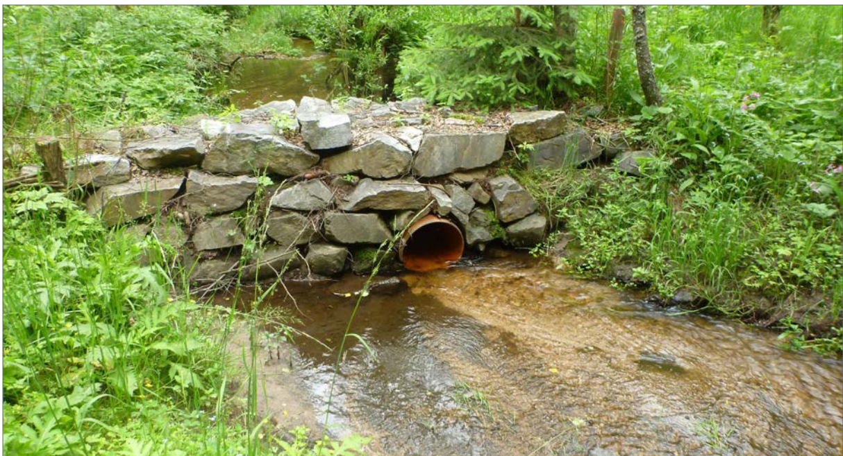
Fig. 185. Semi-permeable dam. Water can flow through this barrier under normal water conditions; however, with increased flow the pipe capacity determines the flow volume. Excess flow rises behind the dam and overflows in the specified direction. To prevent the creation of a migration barrier for trout, the pipe must be placed so the water continuously freely flows through it without a hydraulic jump.
