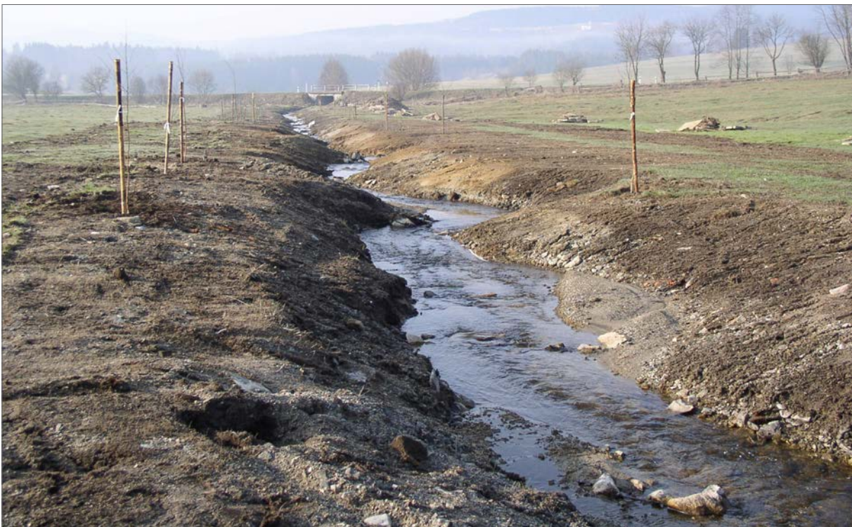
Fig. 197. Restoration process on Zbytinský potok stream and Sviňovická strouha stream. Removing of concrete panels and leaving of a not naturally deep channel on Sviňovická strouha stream in autumn 2004 led to excessive entry of sediment runoff into the main stretch of the Blanice River (a FPM location).
