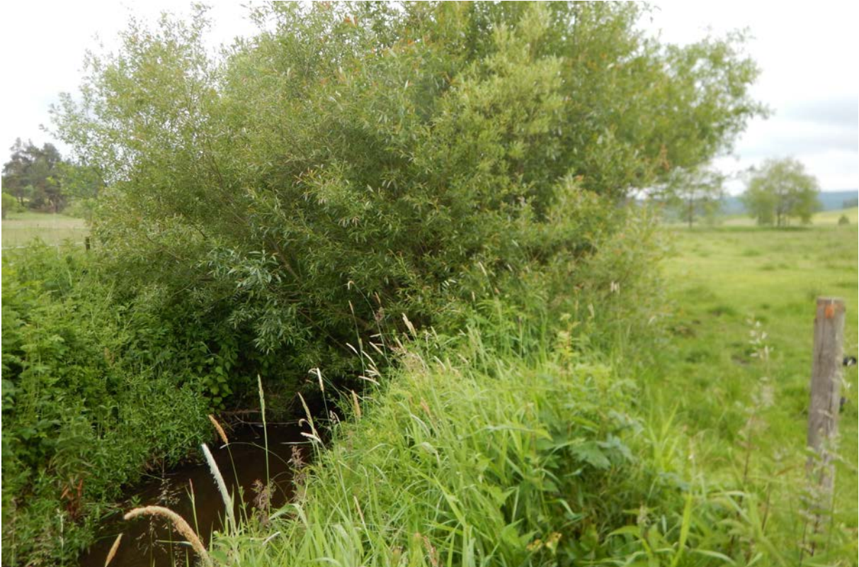
Fig. 261. The same growing fascine bundles with gravel in 2016 as seen from the meadow.
