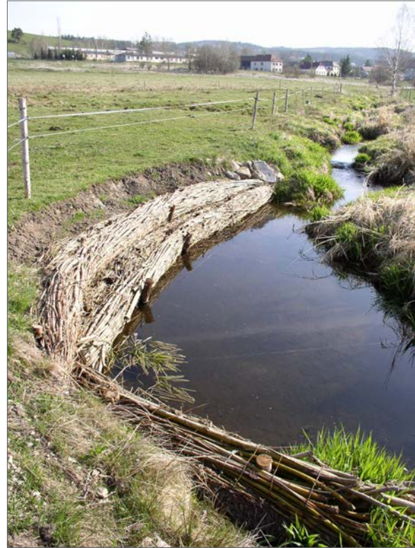
Fig. 199. One metre high ongoing erosion stabilized by a growing fascine bundle in November 2006 (Zbytinský potok stream).
